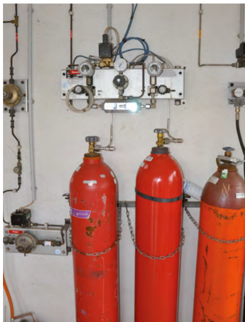
Fig. 18: Compressed-gas cylinders with (acetylene, right) and without (hydrogen, left) the "N" marking
