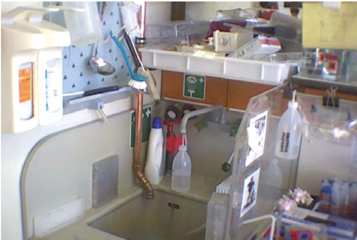
Fig. 32: Emergency eye-wash unit with obstructed access representing a bad example. In the event of an injury, valuable seconds would be lost before assistance could be provided to save the affected eye.
