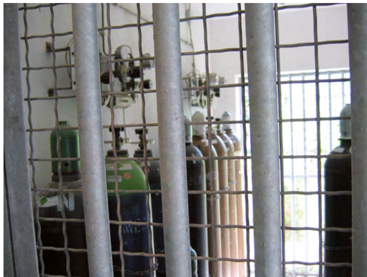
Fig. 17: Gas supply station for laboratory gases outside of the laboratory in a dedicated, well-ventilated room
