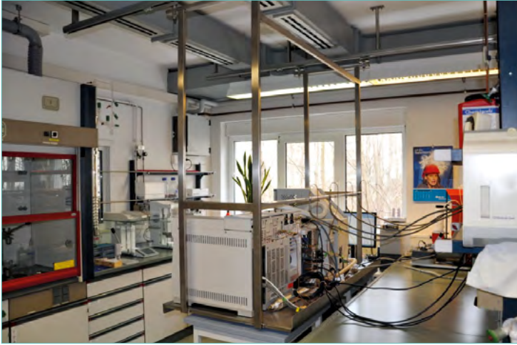
Fig. 9: If no space is available to perform maintenance work behind bulky or heavy equipment, such equipment can also be made mobile. In the figure, a GC/MS device and thermodesorber are installed together on a table that is suspended from the ceiling (observe tensile loads) using a rail system. If necessary, this can then be moved forwards far enough to allow work to be performed behind the device. Mobile tables are pushed under to secure.
